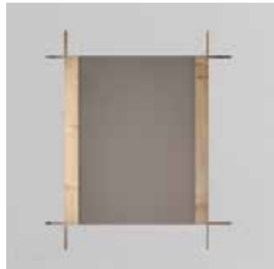
Cut a 225 x 190 x 65 mm hole in the wall and install 2 wooden planks
